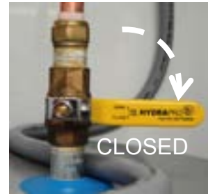
Water Shutoff Valve
