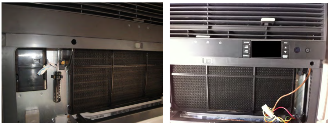
OLD FRIEDRICH 24000 BTU HVAC UNIT
