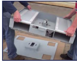
LEM Base Plate being lifted on to LEM Mounting Plate
